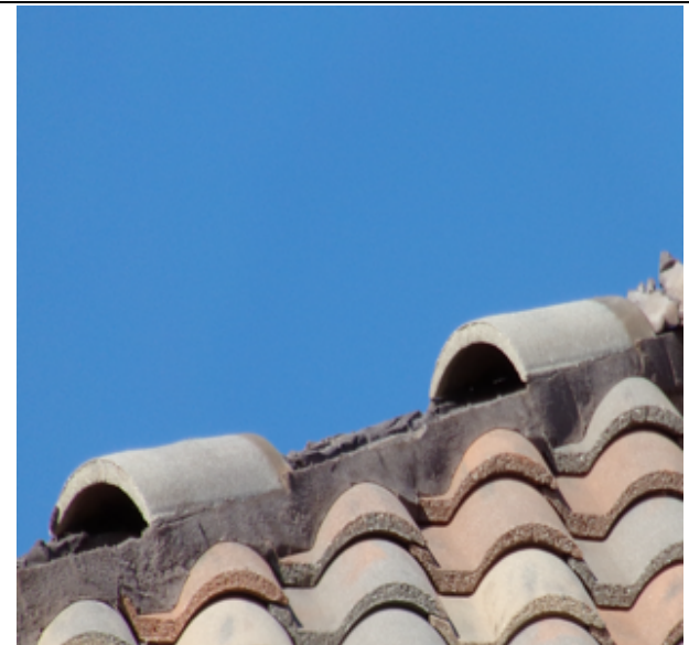
Photo 105: A few mortar-installed tiles were missing along this hip
