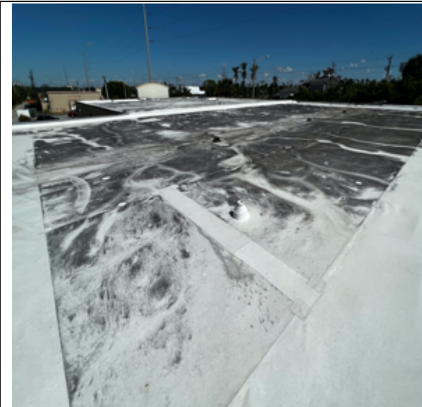
Photo 29: Overview with repaired sections shown as newer/cleaner membrane.
