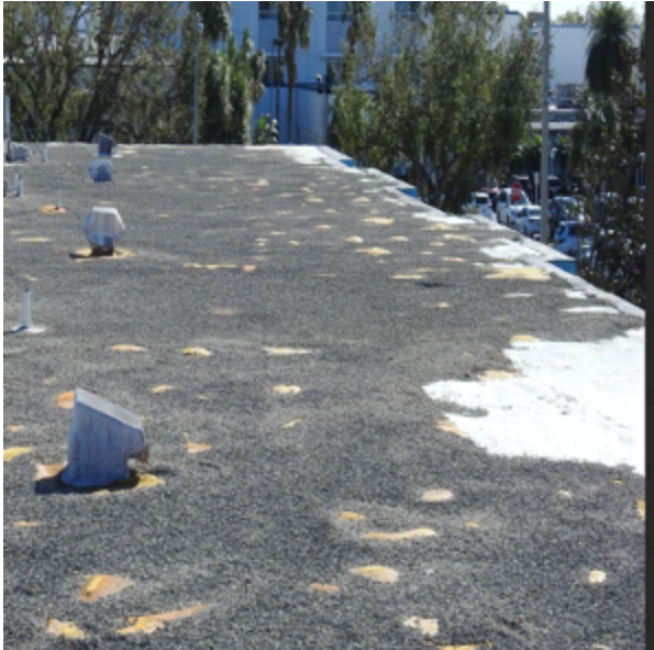
Photo 68: No parapet or gravel stop. Wind scour at all perimeters. Notice widespread blisters are also scoured.
