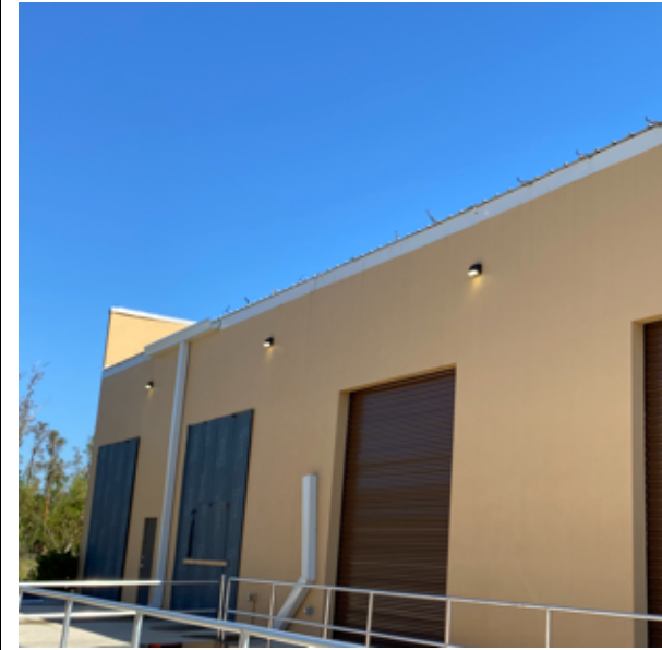
Photo 162: More missing doors and gutters
