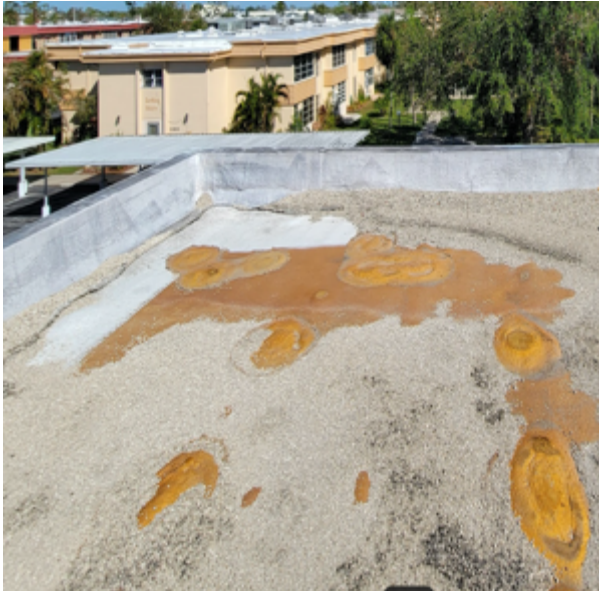
Photo 69: Upwind low parapet typical wind scour of small aggregate.
