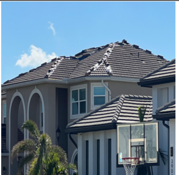
Photo 114: Another tile roof subjected to 110 mph winds, causing dislodged/detached hip tiles.
