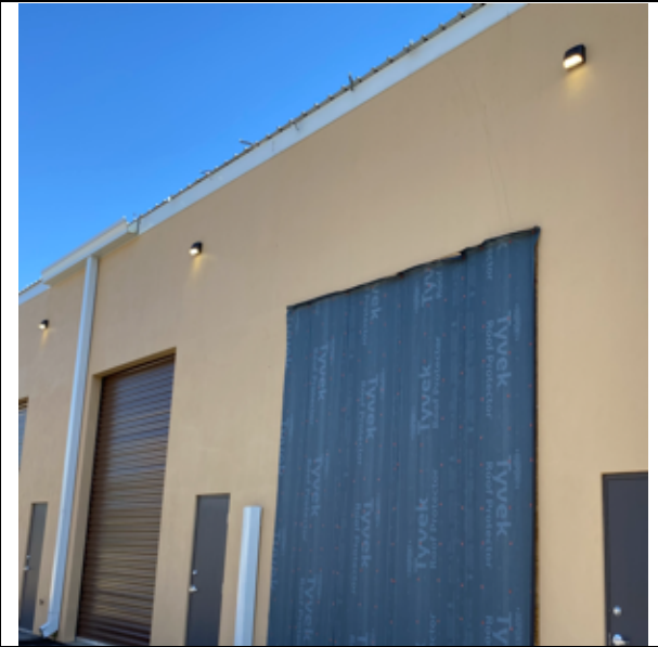
Photo 160: Missing door and gutter
