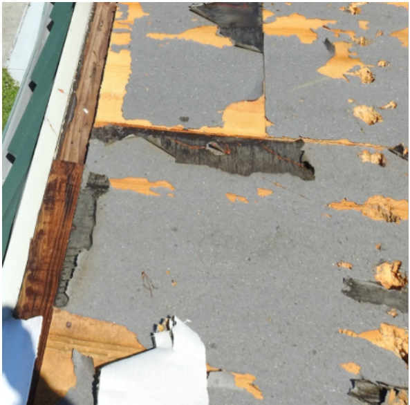
Photo 7: Loss of edge securement was a key factor in membrane blow off.
