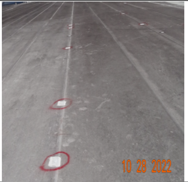
Photo 18: Punctures from air handler parts that became windblown projectiles.
