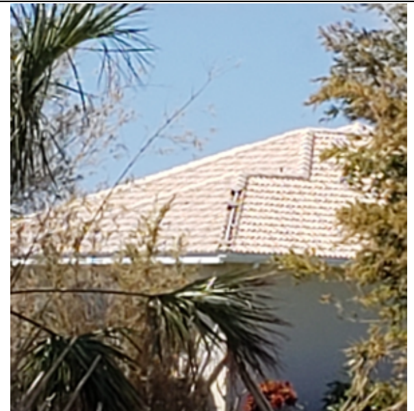
Photo 122: Small area of hip tile missing
