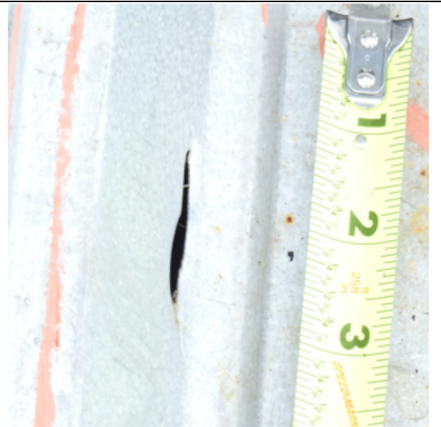
Photo 73: Damage to metal deck from coping hit.
