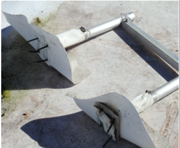
Photo 44: Typical air handler stanchion damage, which often causes punctures, gouges, cuts, or tears in the membrane
