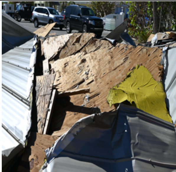
Photo 156: Detached deck and metal roof
