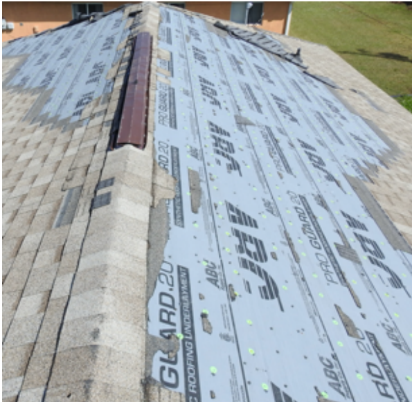
Photo 137: Shingle detachment on a roof constructed in 2022, exposed to 110 mph windspeed.
