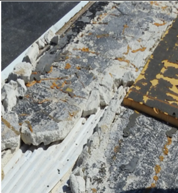
Photo 10. LWC damaged and metal edge missing.
