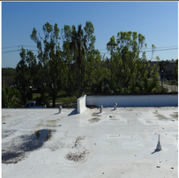
Photo 34: Intact edges indicate that much of the roof was relatively undamaged.
