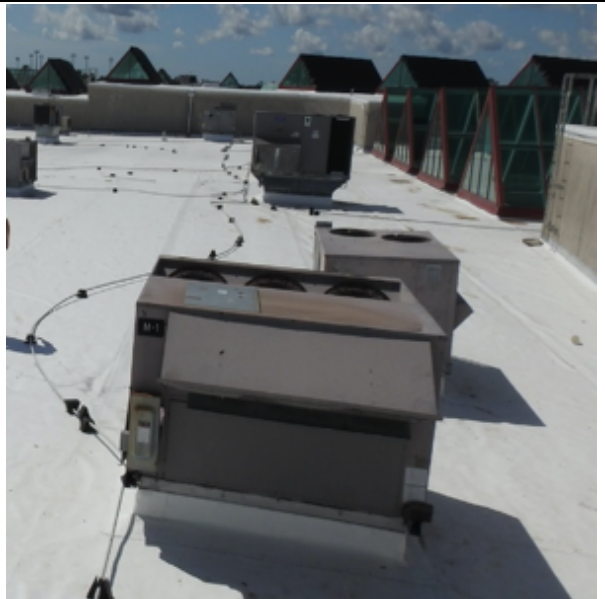
Photo 53: Loose lightning arrester wire
