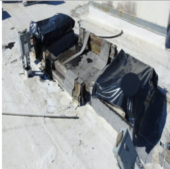
Photo 41: Air handling unit displaced
