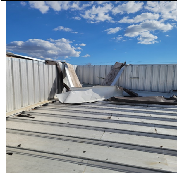
Photo: Damaged edge metal and 1/2 inch plywood sheet
