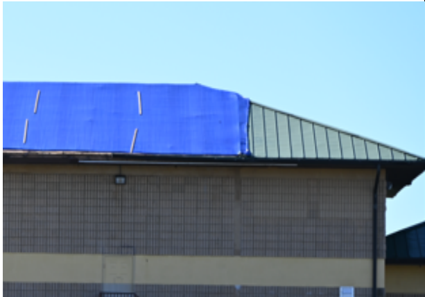
Photo 88: Tarps cover most of the roof
