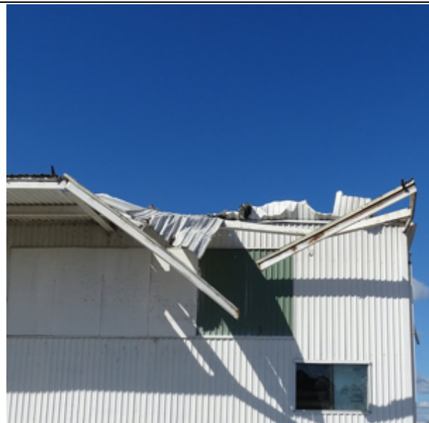
Photo 94: Overhangs are vulnerable, more bracing was needed, 110 mph winds.
