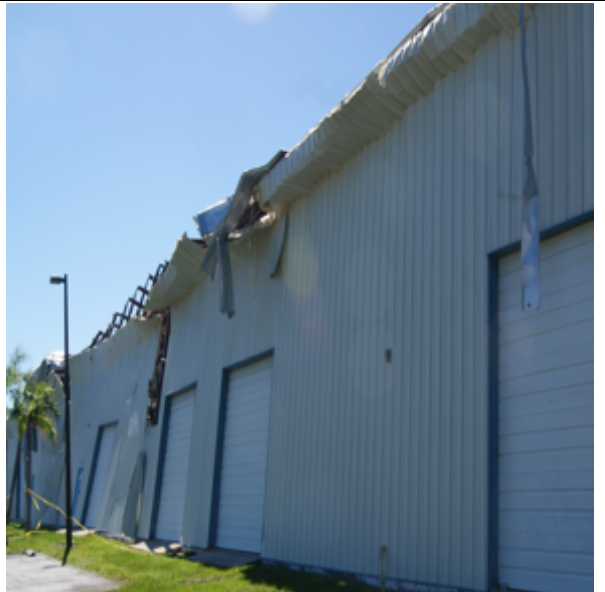
Photo 84: Doors resisted the winds.
