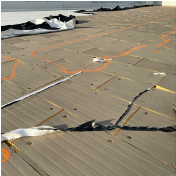
Photo 13: Near total blow off of a mechanically attached single ply system. It originated at a roof corner where ground-floor window damage caused a breach in the metal deck and pressurized the roof.
