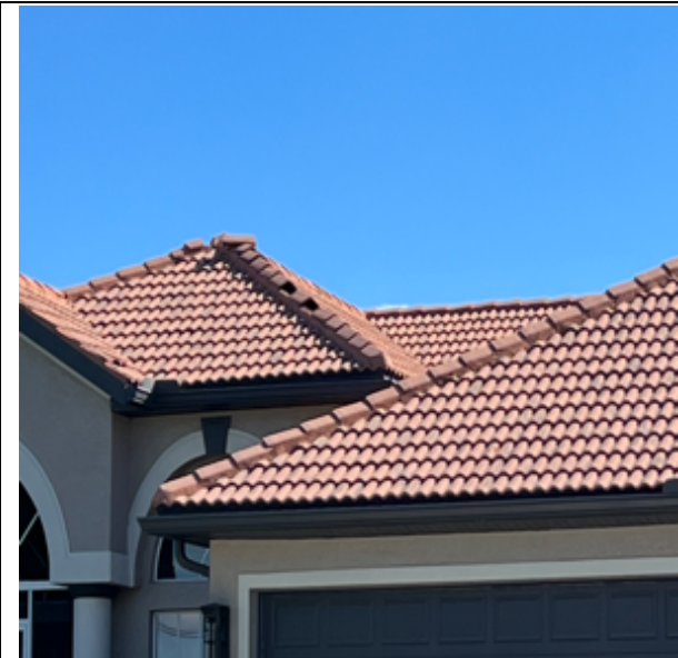
Photo 113: SW 39 th Ave Cape Coral A tile roof subjected to 110 mph exhibited some hip damage.
