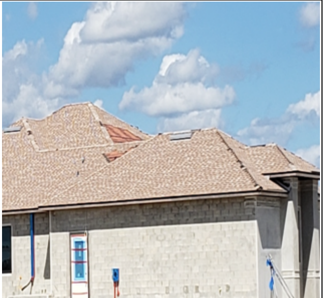
Photo 136: Hip and ridge damage that appears to have spread
