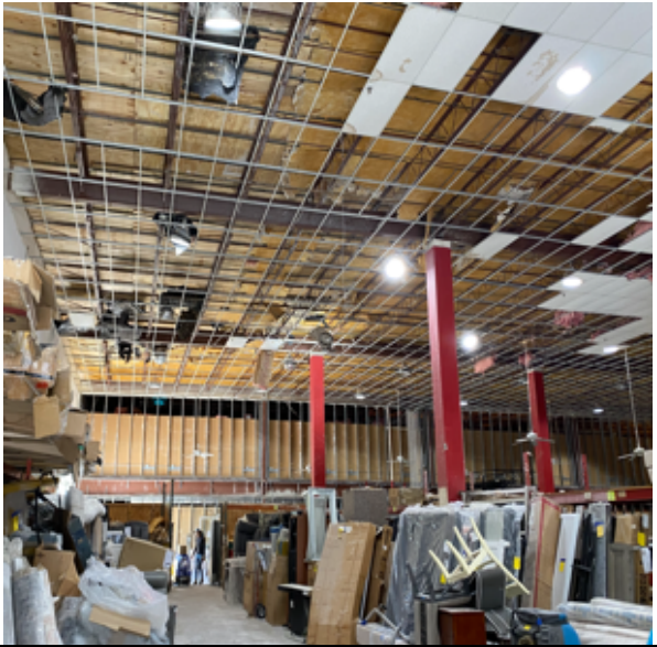
Photo 62: Significant interior and product damage
