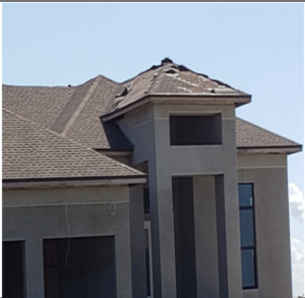
Photo128: Some damage on high roof
