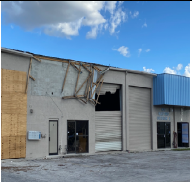
Photo 75: Decorative protective entrance cover completely missing
