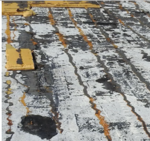
Photo 11: Limited low-rise foam resulted in inadequate wind uplift resistance.
