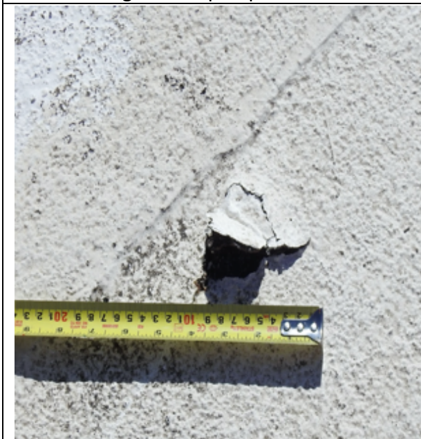
Photo 42: Cut from debris
