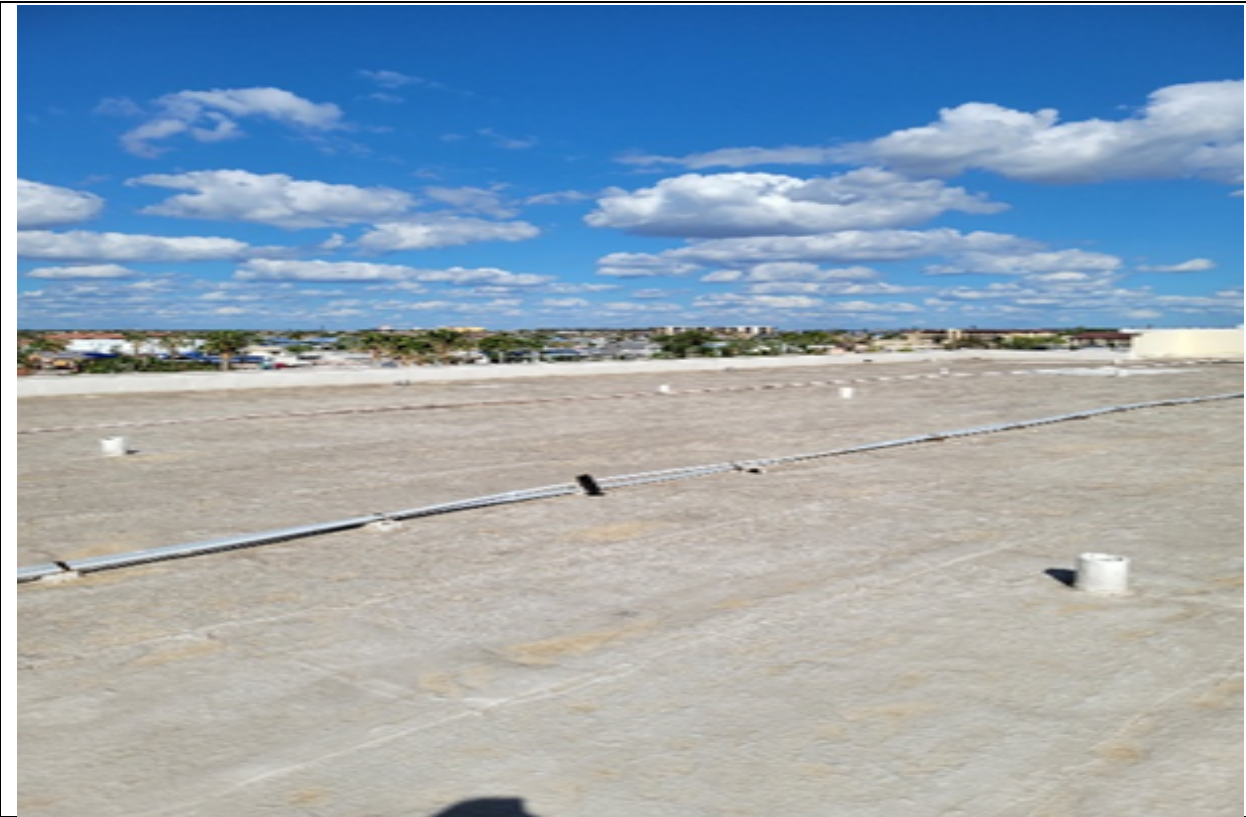
Photo 45c: The rest of the roof was not damaged
