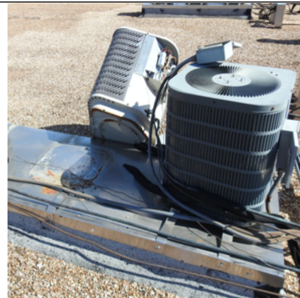
Photo 58: Damaged air handling unit
