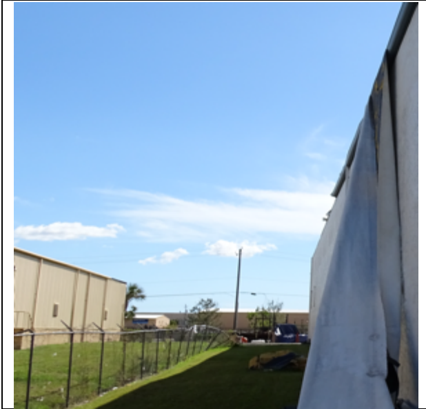
Photo 166: Gutters missing on windward (front) side of two adjacent buildings
