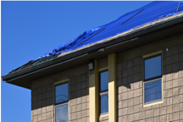
Photo 87: About half this metal roof may have been damaged
