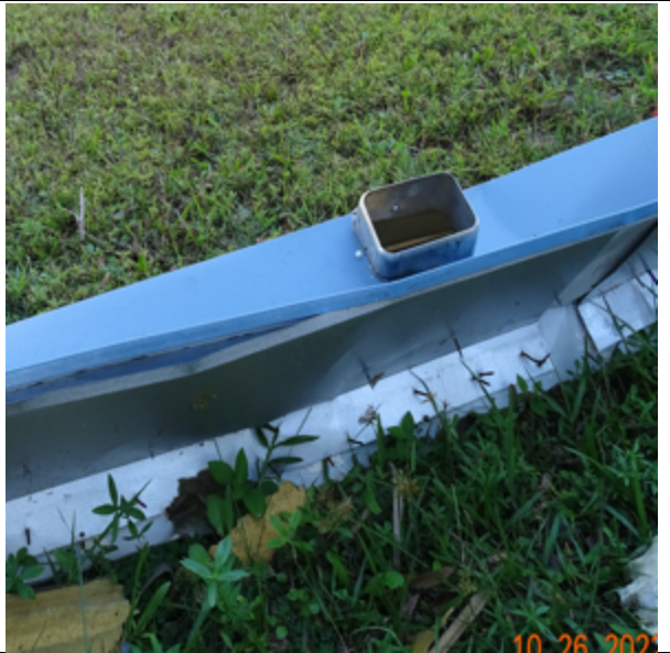
Photo 167: Detached edge metal and gutter
