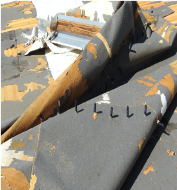
Photo 8: Close fastener placement along the perimeter appeared to be intended as a peel stop but attachment to lightweight concrete (LWC) deck was inadequate.
