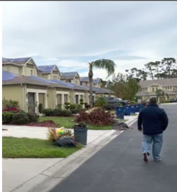
Photo 145: The opposite side of the street had many tarped roofs. Residents reported that houses on this side of the street had not been reroofed. They are likely original roofs installed around 2005.
