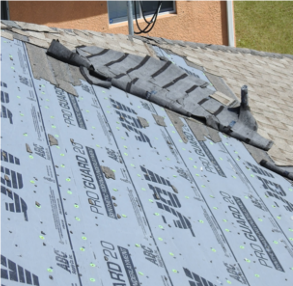
Photo 138: Note that the shingles were still bonded together, exhibiting low loss of sealant strip adhesion. Inadequate nailing may have contributed to detachment.
