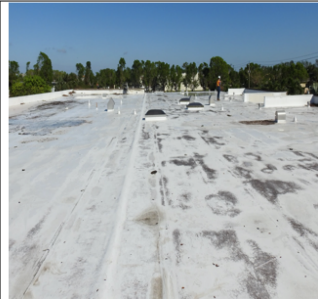
Photo 33: An overview shows that the field of the roof appears largely undamaged.
