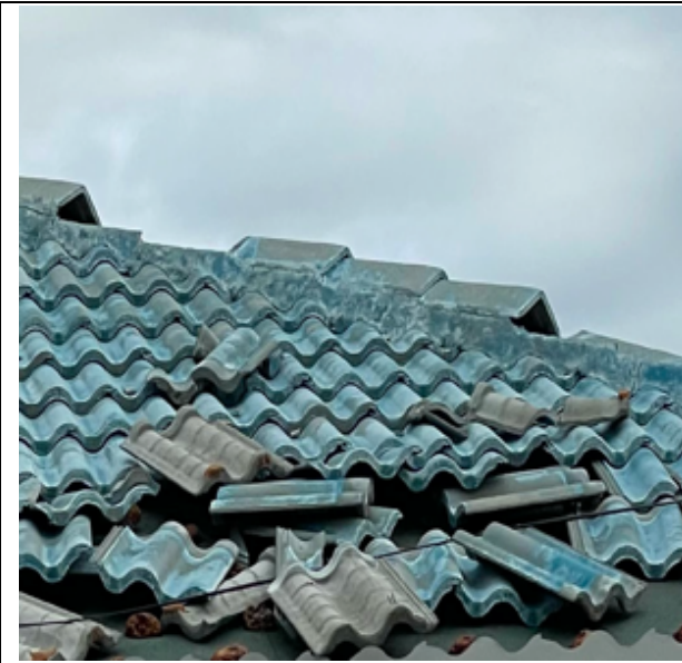
Photo 111: Older system subjected to 110 mph winds, resulting in dislodged and detached tile
