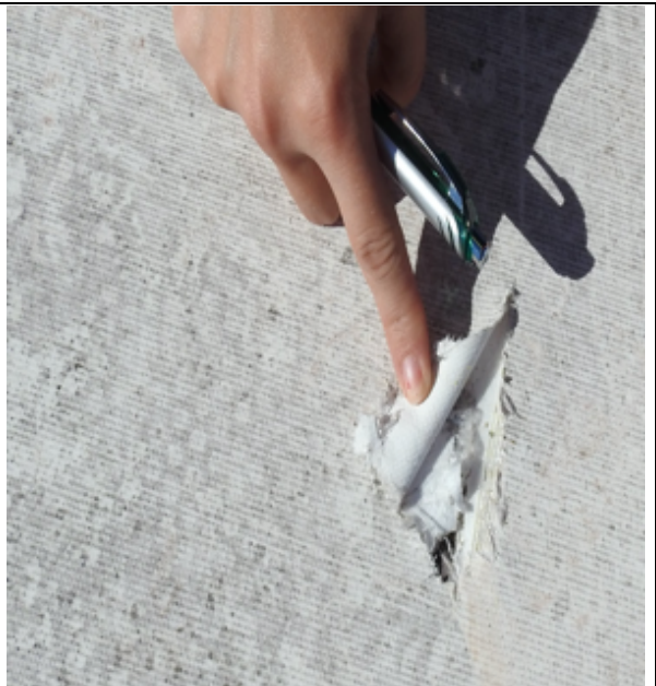
Photo 40: A typical membrane tear or cut from the traumatic impact of either a windblown projectile or wind-propelled object tumbling over the roof surface.
