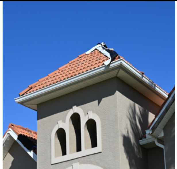
Photo 118: Tile missing from high hip
