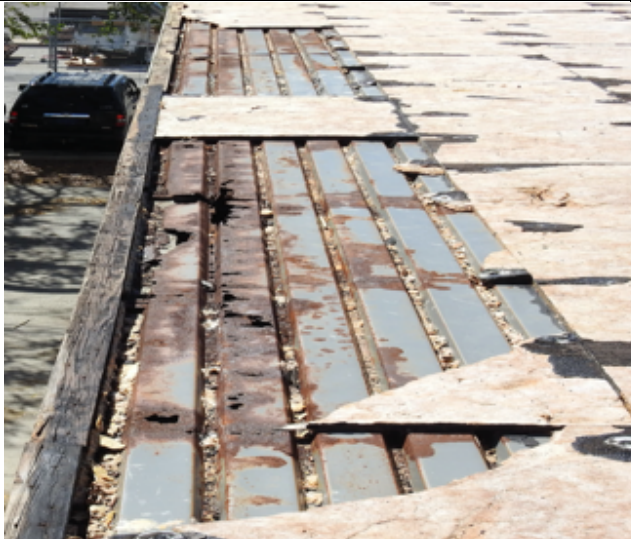
Photo 48: Rusted deck main source of blow off
