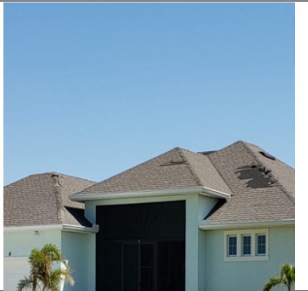
Photo 132: Some field of roof damage
