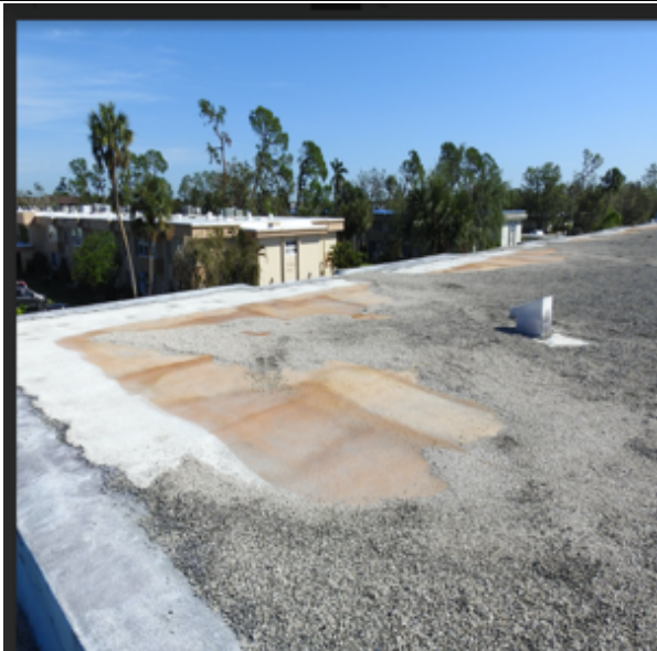
Photo 66: Foam is intact, significant scour
