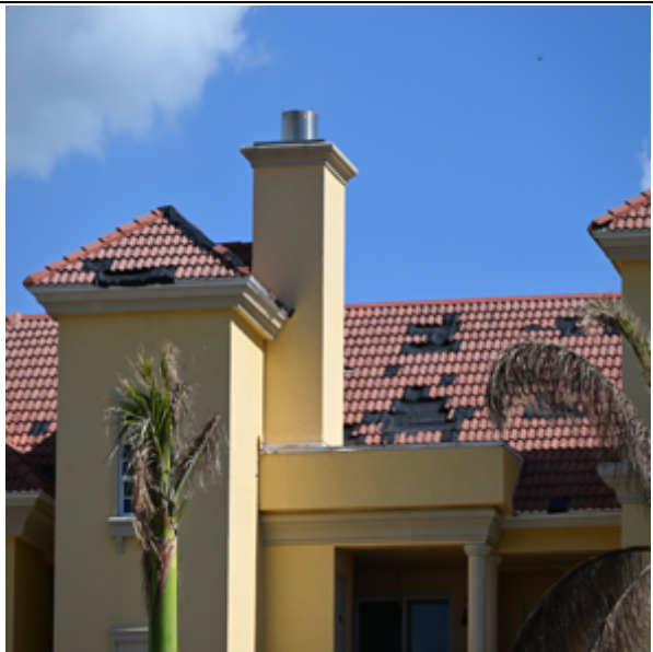
Photo 110: Random impact damage from windblown projectiles; underlayment intact.
