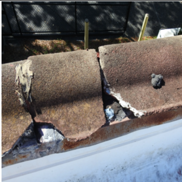
Photo 36: Damaged tile, from windblown projectile impact or wind-induced vibration.
