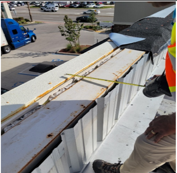
Photo: Missing coping increasing risk of water infiltration
