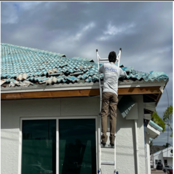
Photo 112: Area of damage, along roof edge
