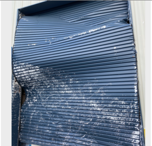
Photo 77: Another damaged door
