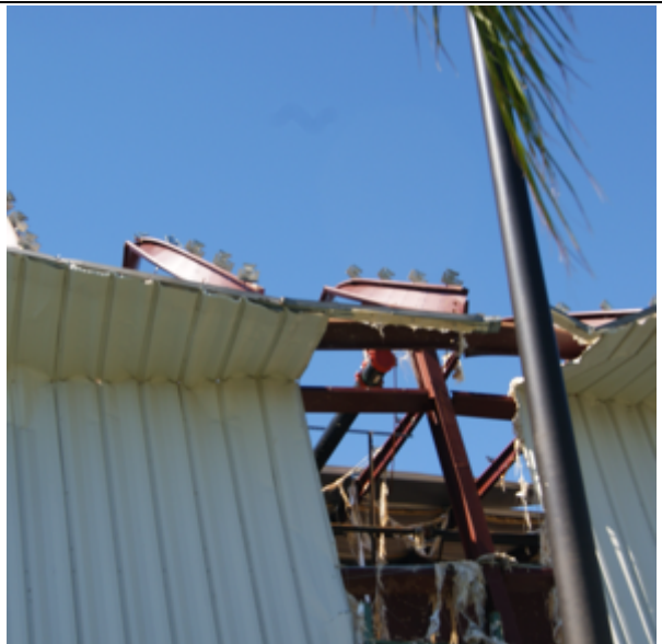
Photo 82: Wall is breached
