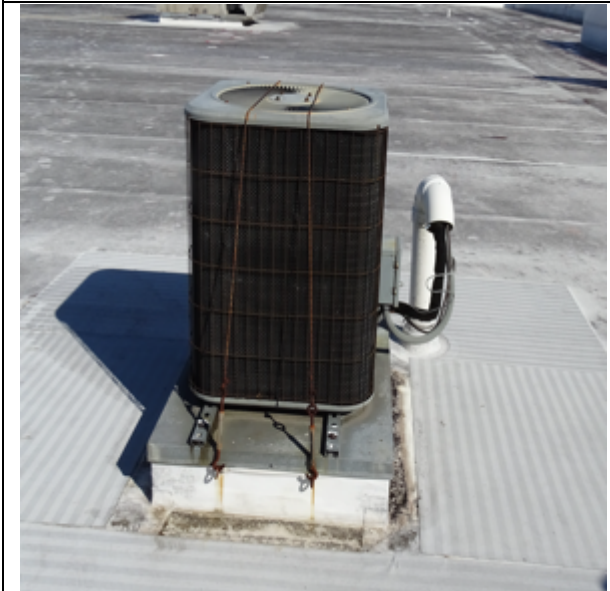
Photo 19: A secure air handler still attached.
