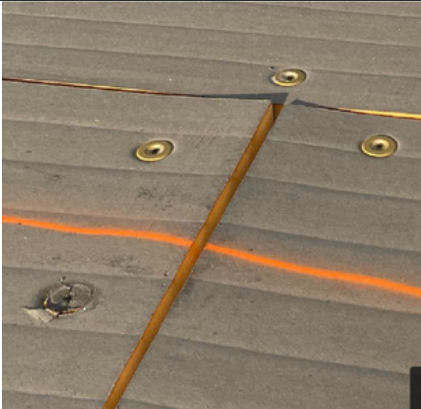
Photo 15: A fastener with a good weld and fasteners with incomplete welds.
