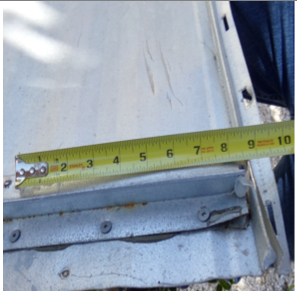
Photo 97: Hip flashing failure due to rivets being spaced at 30" O.C. to cleat.
