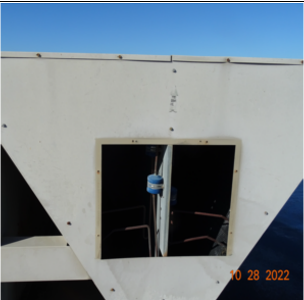
Source of much of the roof damage i.e., when inspection panel detached it became a windblown projectile with sharp corners.
