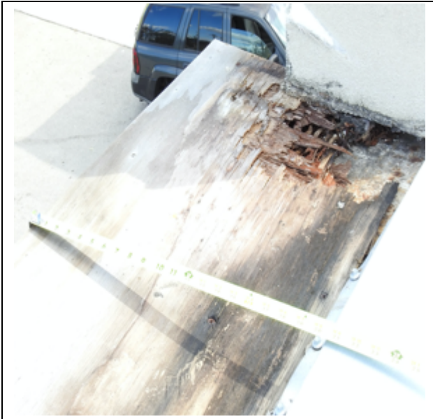
Photo 72: Top of rotted parapet, inadequately fastened coping
