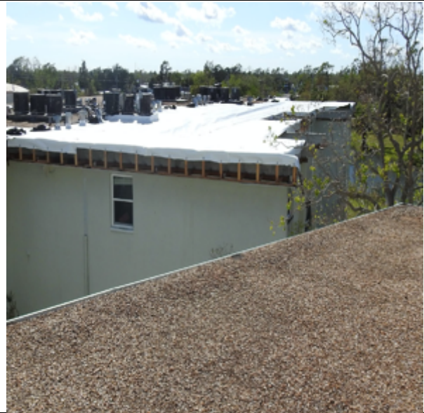
Photo 57: Another roof section with a temporary roof. Note no parapet or gravel stop. Also, soffit damage.
