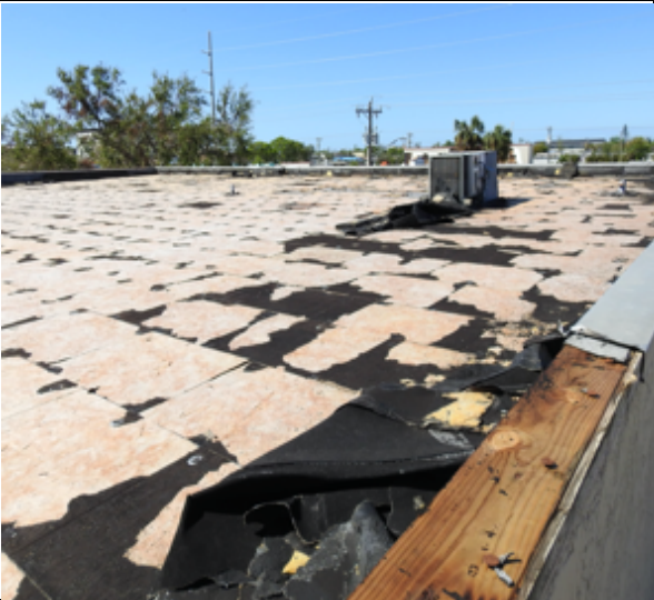
Photo 47: Some parapet damage
