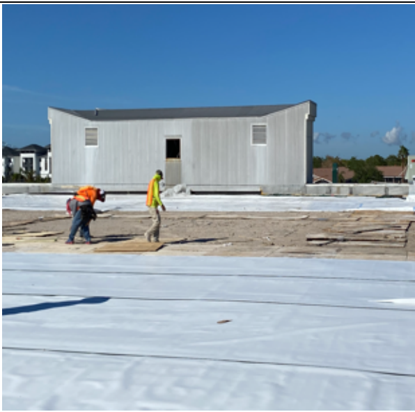
Photo 61: Temporary(?) Roof installation. Plywood being placed between membrane and lightweight concrete, both to separate and provide a safe (?) walking surface.
