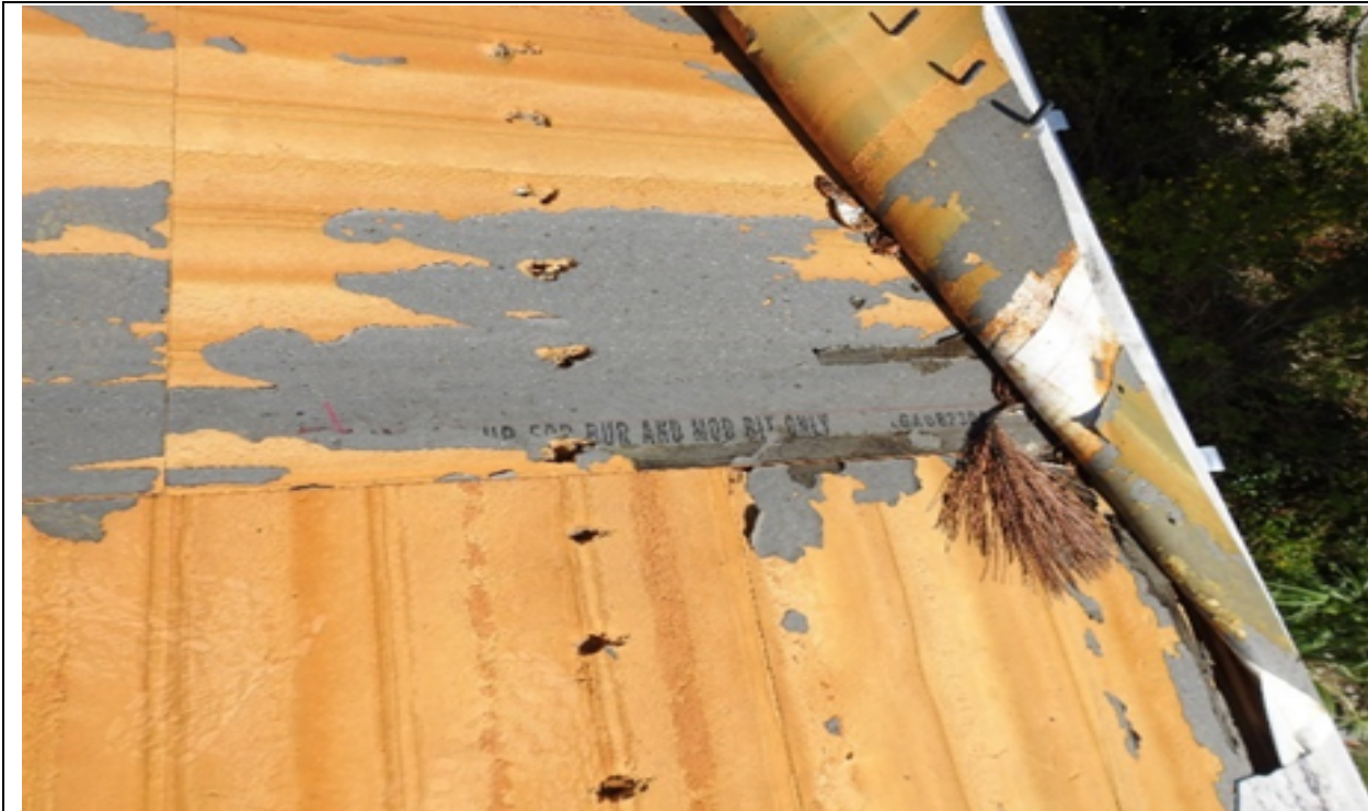
Photo 13: Improper insulation used. Insulation was marked to be used only with BUR and Mod Bit membranes
