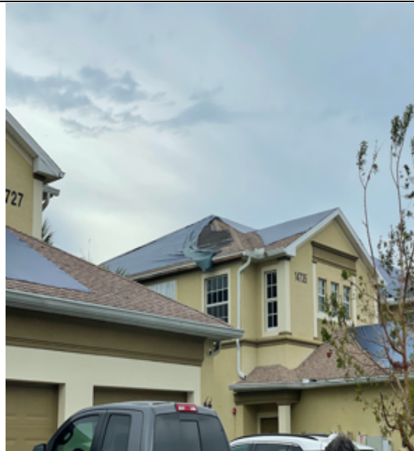
Photo 146: These asphalt shingles were detached from roofs on the west side of the street.
