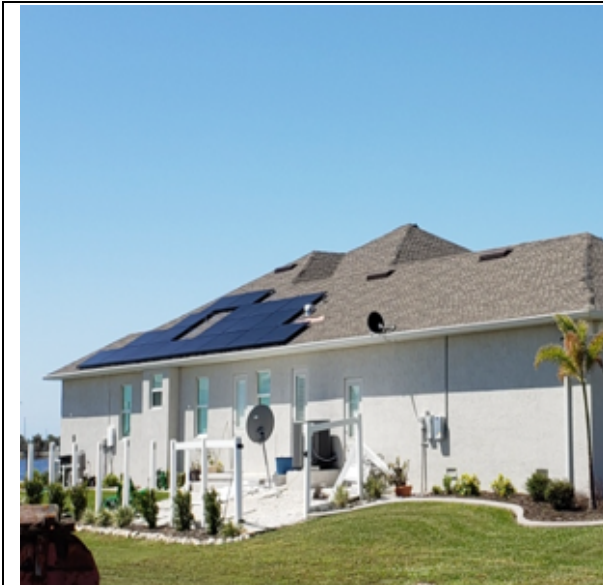
Photo 133: Solar array undamaged
