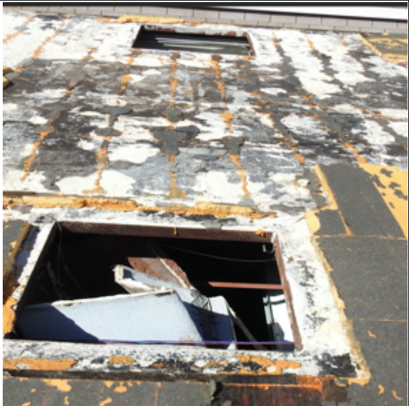
Photo 12: Sky lights became detached along with insulation and AHU's
