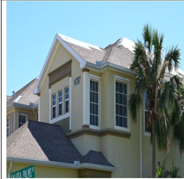
Photo 147: The roof had ridge damage and some field damage
