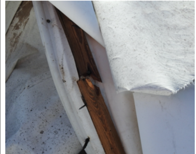
Photo 43: Edge damage like this may allow water intrusion through openings between roof membrane and deck.
