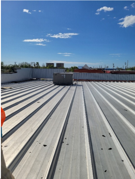
Photo: The right of the roof was mostly undamaged
