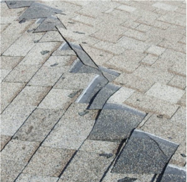
Photo 140: Hip shingles were inadequately adhered.
