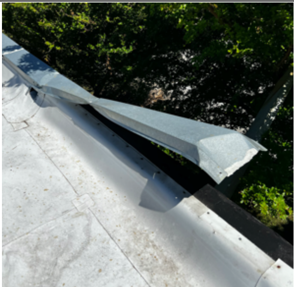
Photo 30: Metal coping partial detachment.
