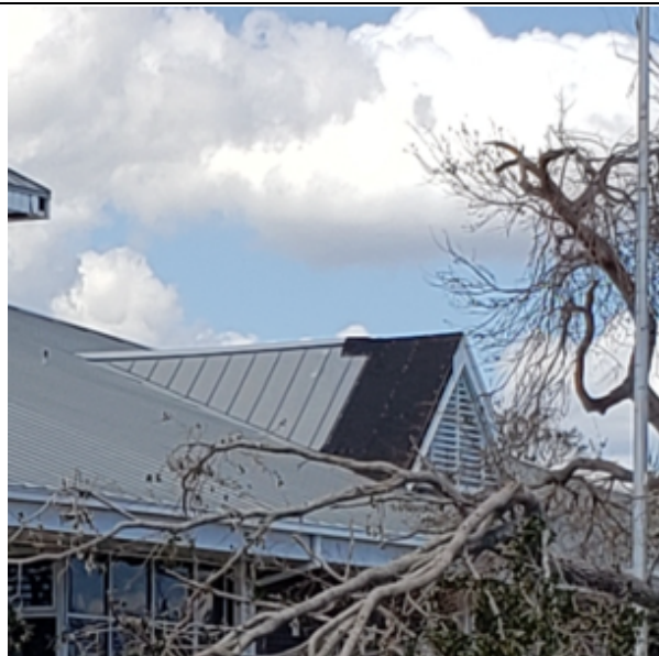
Photo 93: Damaged roof in 130 mph windspeed. Inadequate edge fastening
