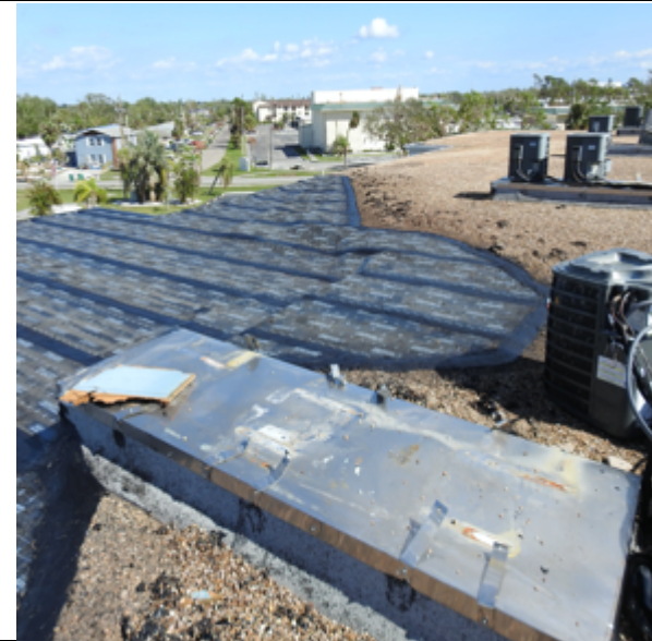
Photo 56: Temporary patch in corner
