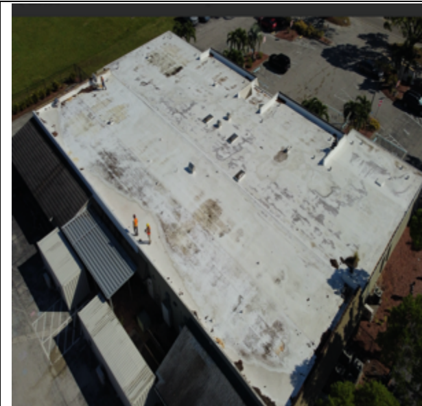
Photo 37: A drone view of the Pace Center roof shows the field largely undamaged.
