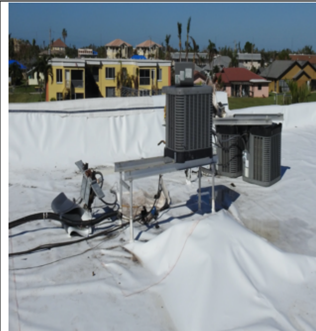
Photo 41: Typical air handler damage from storm winds blowing units from stands and/or curbs.
