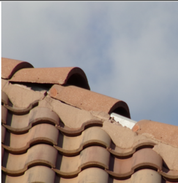
Photo 106: This was a frequent scene with a few hip tiles not contacted with SPF
