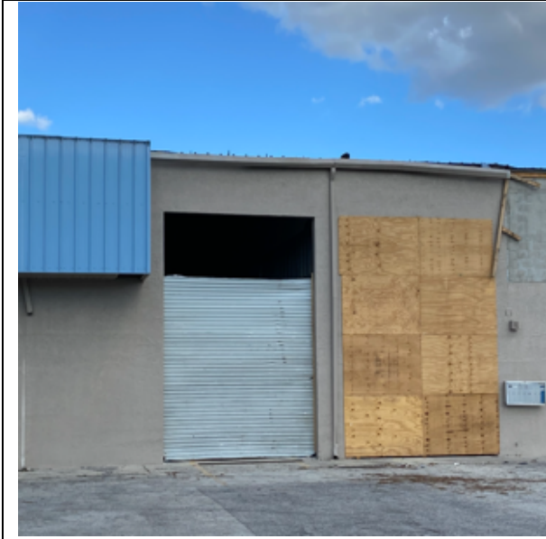
Photo 76: Intact entrance cover, door damage
