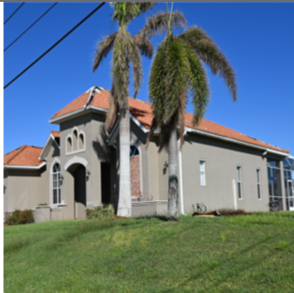
Photo 117: Typical missing tile on hip
