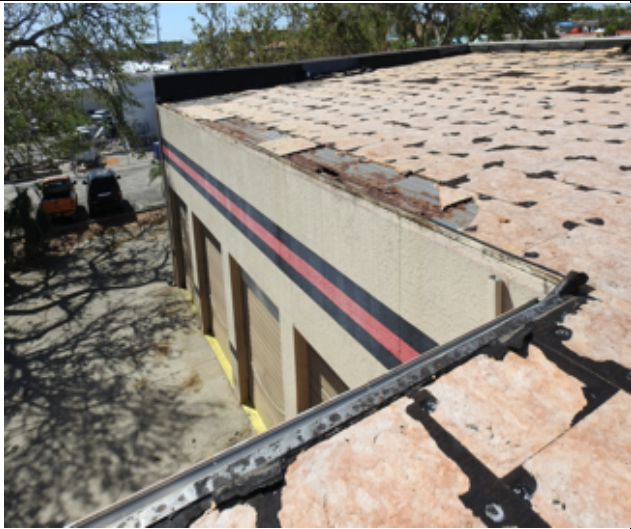
Photo 46: Adhered Mod Bit damage
