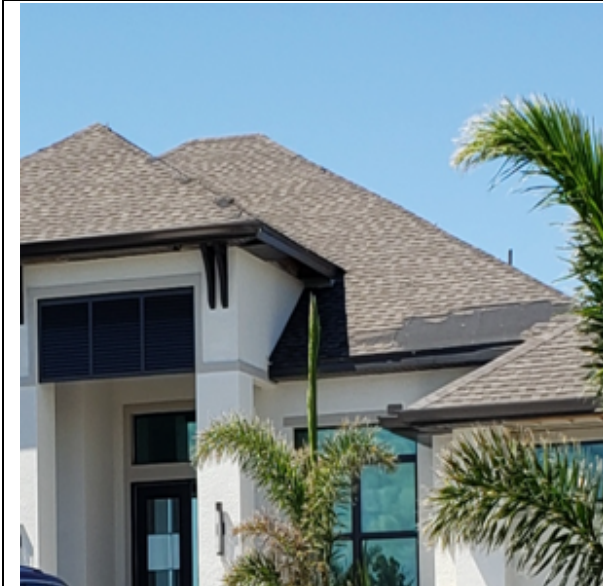
Photo 135: Unusual damage location on hip and eave
