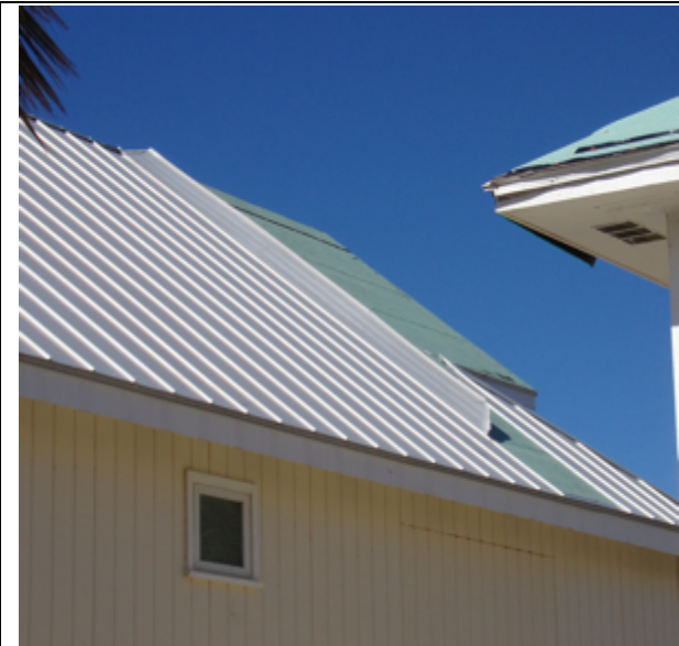
Photo 95: Panels missing on rake edge
