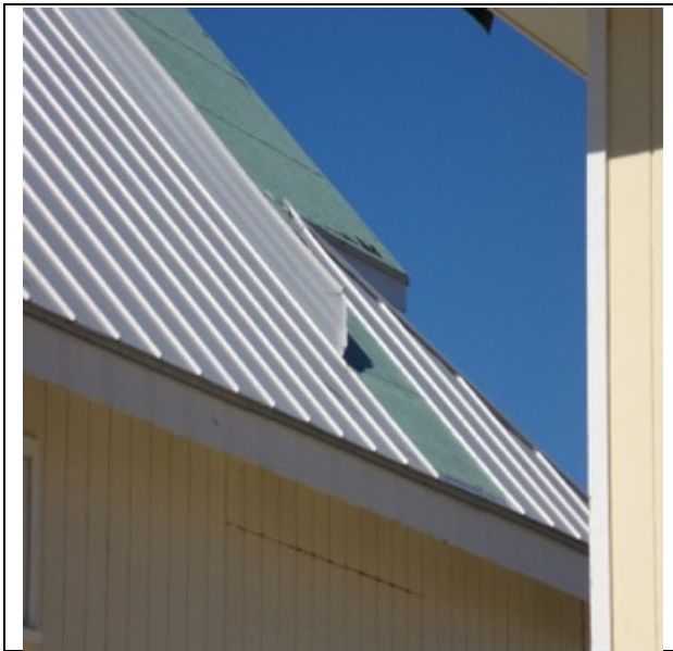
Photo 158: Edge metal damage resulting in loss of panels
