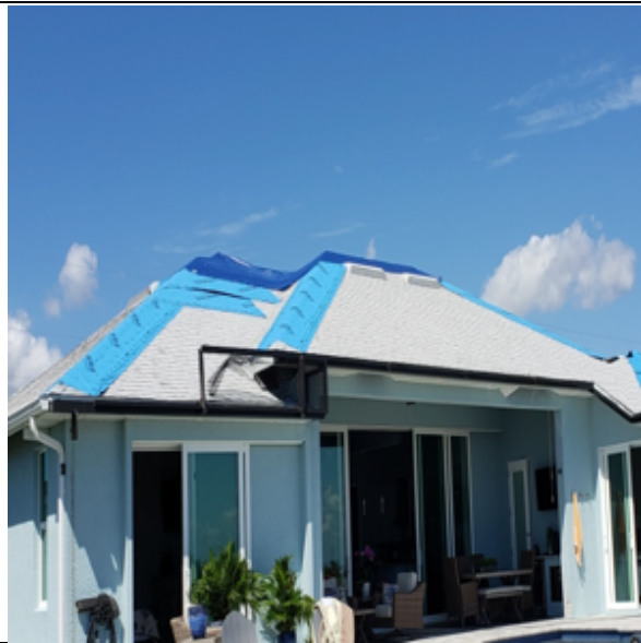
Photo 131: Hip and ridge damage
