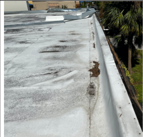
Photo 31: Extensive metal coping detachment left openings for water intrusion between membrane and deck.
