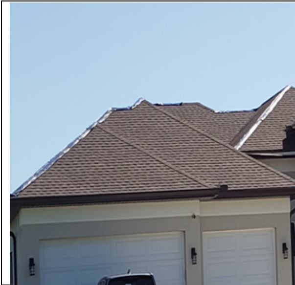
Photo 127: Ridge and hip damage
