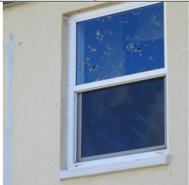
Photo 59: Missing down spout, and debris damaged window
