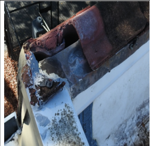
Photo 35: Damaged edge and tile, apparently from windblown projectile impact.
