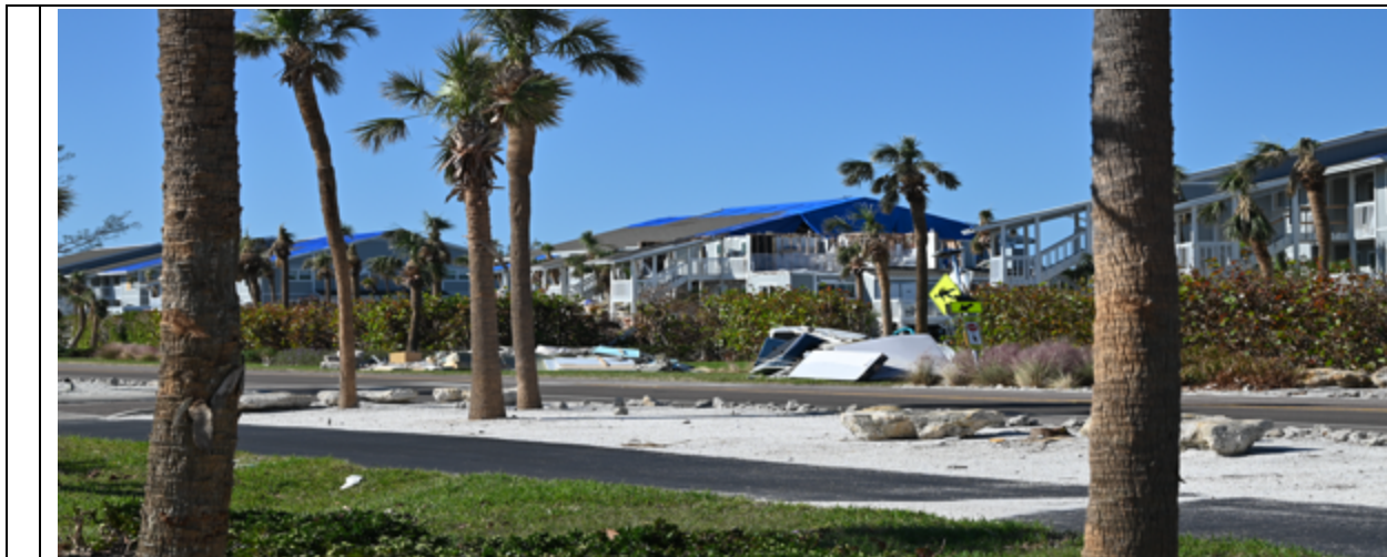
Photo 153: Difficult to diagnose damage initiation, but ridges and rake areas appeared likely to be a primary source of damage initiation.
