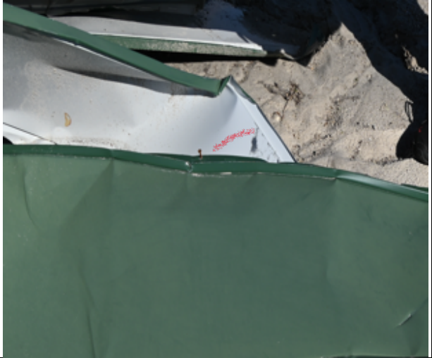
Photo 90: This tiny fastener did not hold the metal
