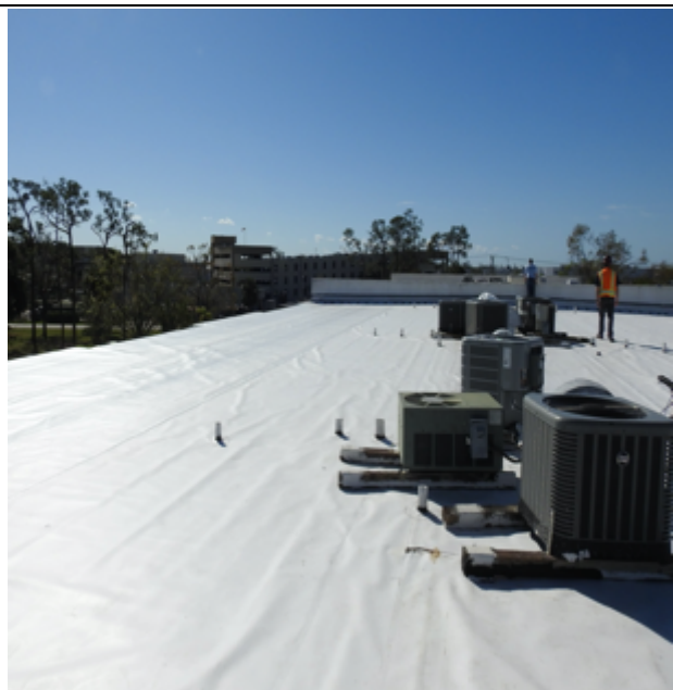
Photo 43: Roof section with temporary recover
