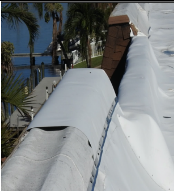
Photo 42: Some parapet damage.
