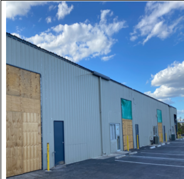
Photo 74: Metal roofed building with minimal roofing loss, with gutter damage
