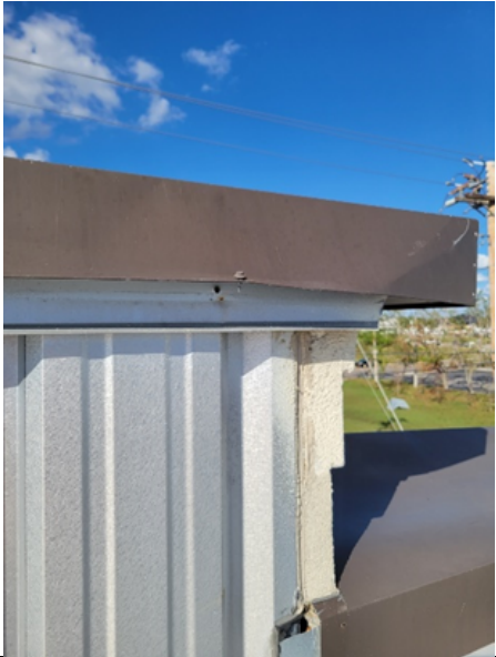
Photo: Fastener pulled out of the coping
