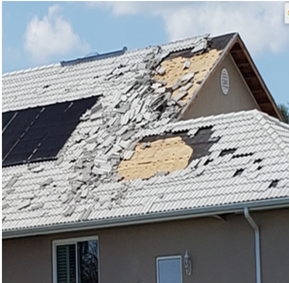
Photo 108: This is an extreme case of tile and underlayment detachment. Tiles were nailed.
