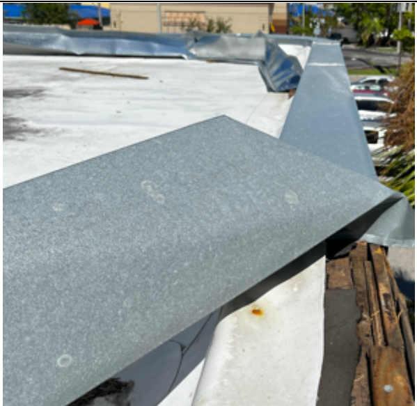
Photo 32: Lack of edge metal fasteners caused coping to have inadequate wind resistance and contributed to detachment.
