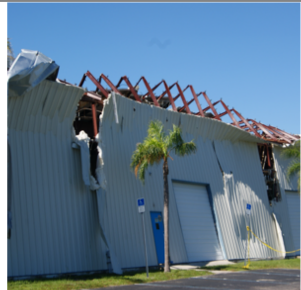
Photo 81: This wall faces Northeast, where the greatest wind speed gust in Hurricane Ian is likely.
