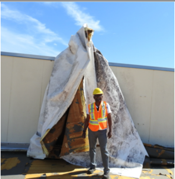
Photo 6: A large piece of membrane was left hanging over the roof edge.
