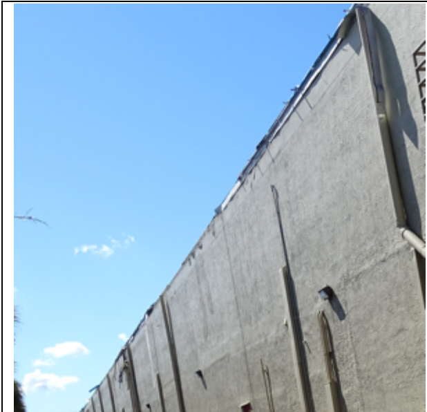
Photo 164: Missing gutters and downspouts
