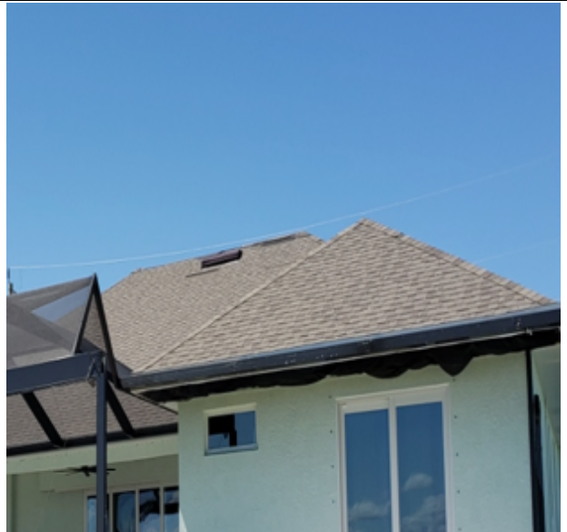
Photo 130: Small amount of hip and ridge damage.
