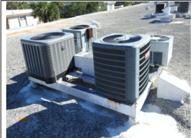
Photo 70: Intact air handlers
