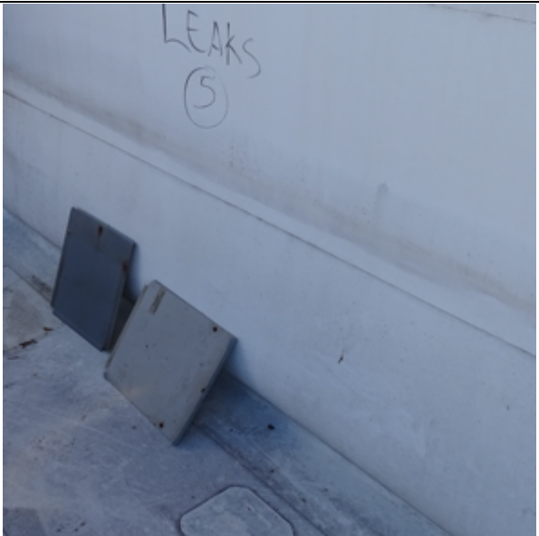
Photo 23: Detached metal panels that were dislodged and created many cuts in the membrane on this roof.
