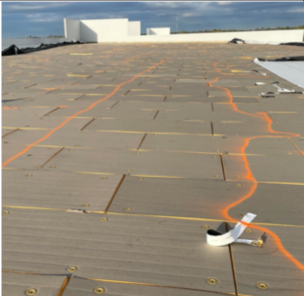
Photo 14: There were large areas where the induction welds to fasteners were completely missed or poorly done, making them more vulnerable to blow off.
