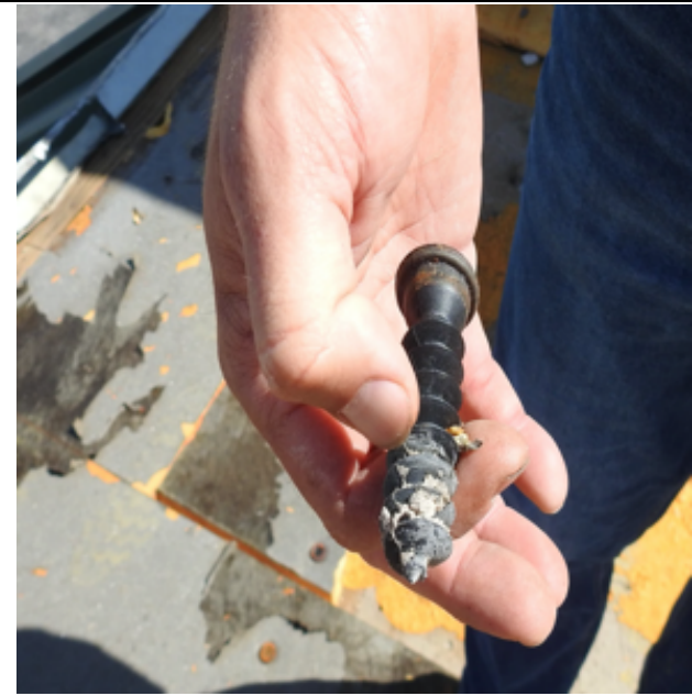
Photo 9: Fastener was not adequately embedded in LWC
