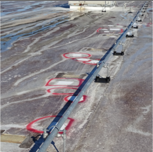
Photo 24: Pipe was moved by wind, tearing the membrane.
