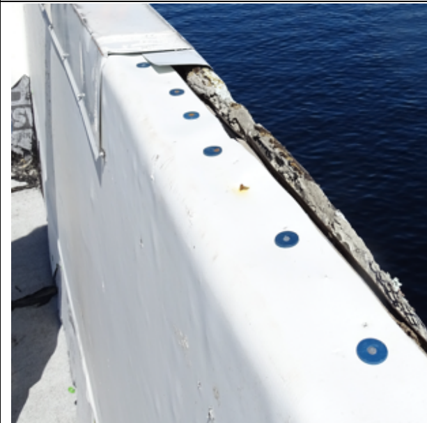
Photo 28: All three buildings had significant coping and edge metal detachment.
