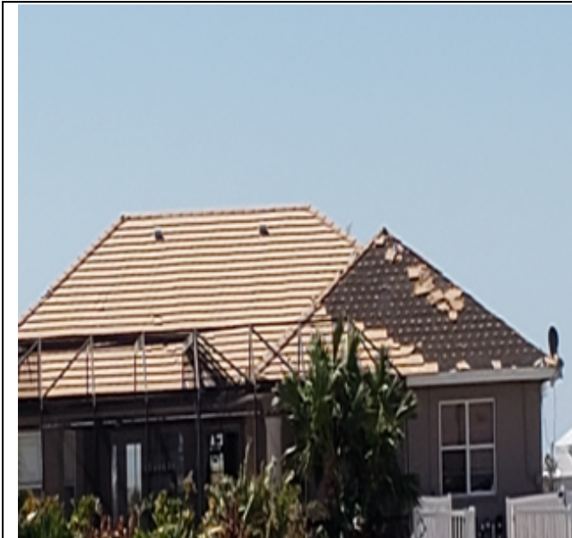
Photo 121: One example of tile loss. Cause not determined.
